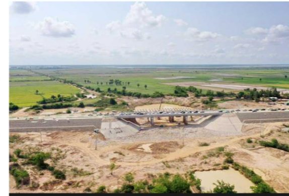
The construction of National Road 11 connecting Peam Ro district to National Road 1 in Prey Veng province in May last year. PUBLIC WORKS MINISTRY
